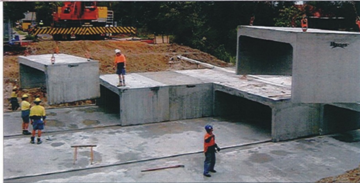
Council workers install the large box culverts measuring 15-metres wide by 1.5-metres high.
